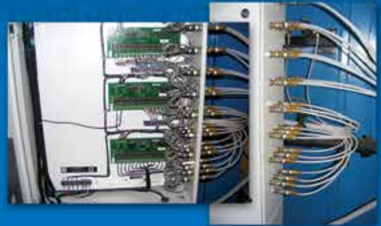
Pressure Transducer Monitoring Lines and Data Acquisition Control System
