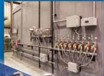
Vacuum Piping System w/Pressure Transducer & Thermocouple Jack Panel
