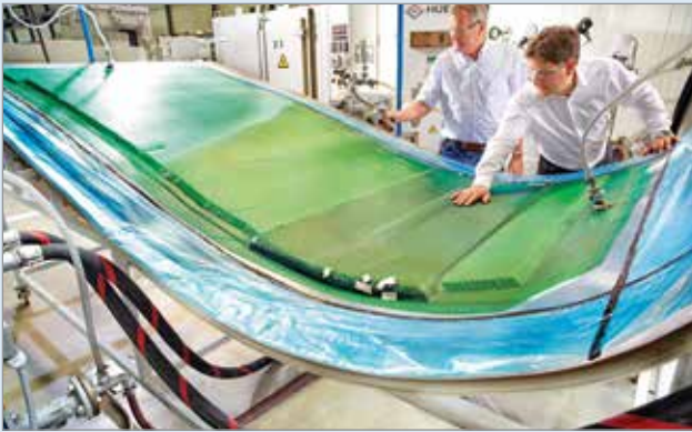
1 Covestro tested its latest polyurethane resin, glass fiber reinforcements and infusion setup, including injection equipment, prior to the spar cap demonstration. Source (all step photos) | Covestro
