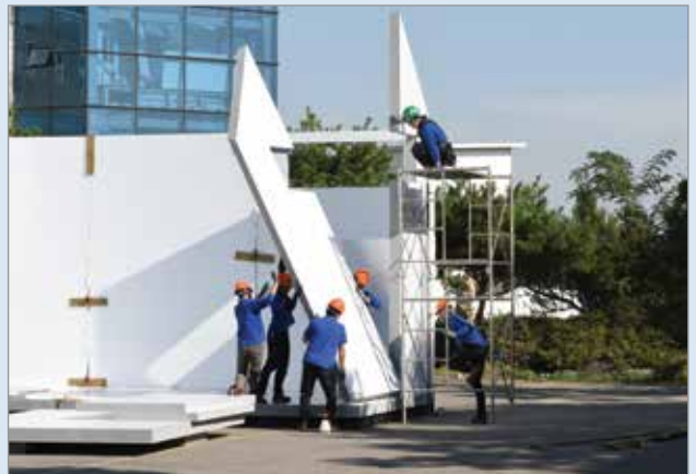
4 Adjacent panels were then bonded to each previous panel, glued along edges and to the floor, moving around the perimeter of the house until the walls were constructed.
