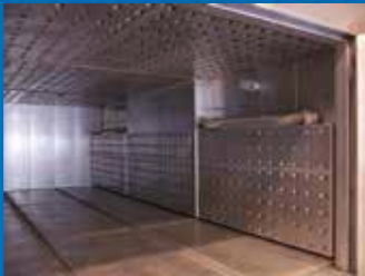
Interior Supply and Return Ducts with Interior Lighting
