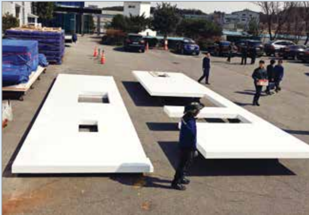
2 Panels were readied to be flat-packed into a standard shipping container for transport to the construction site.
