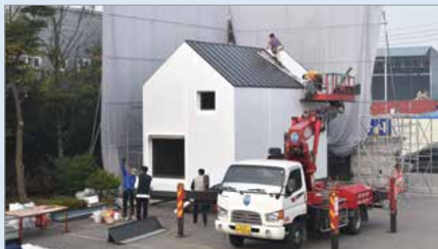
7 By day four, windows and door installations were completed, as were interior plumbing and wiring, and a zinc roof system was in progress.
