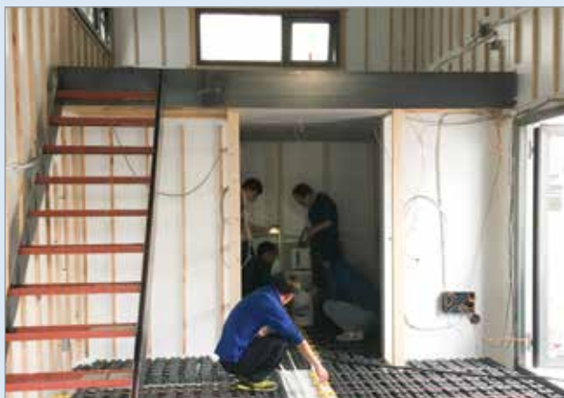
6 On day two, window and door installations had begun and the floor heating system was installed.
